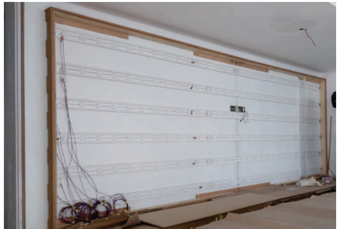
THESE LEDS CAN BE PULLED OUT FROM THE SIDE IN FUTURE
